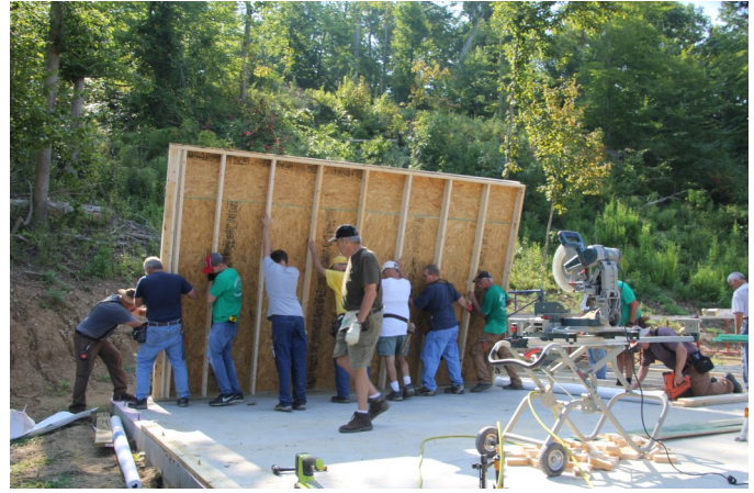
Members of FBC's Baptist Builders work to set the very first wall in the Justin Butcher Memorial Lodge at Seneca Lake last month. The new lodge is expected to open next spring.
